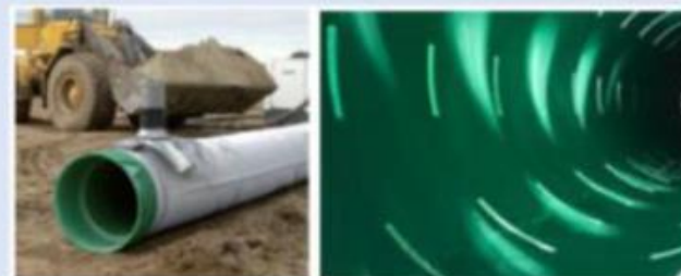
Figure 10: Drainage and horizontal subsurface drainage pipes (source: WSVN)
